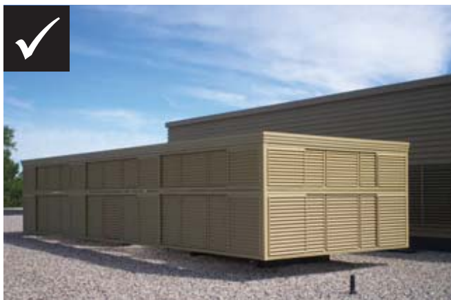
Screened rooftop equipment
