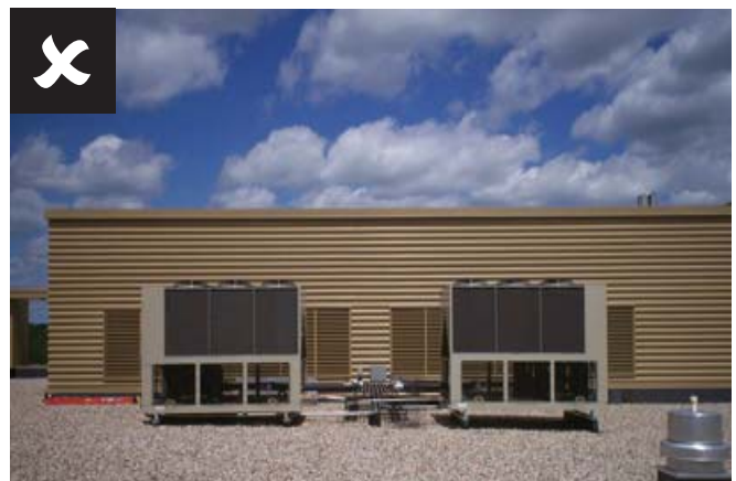
Unshielded roof-top equipment
