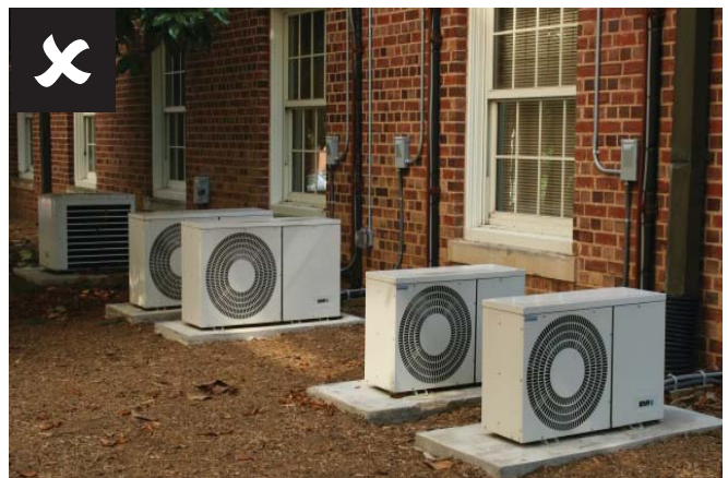
Unshielded ground-level equipment
